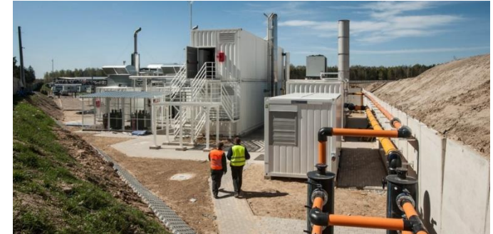
Heat recovery system (HRS)
